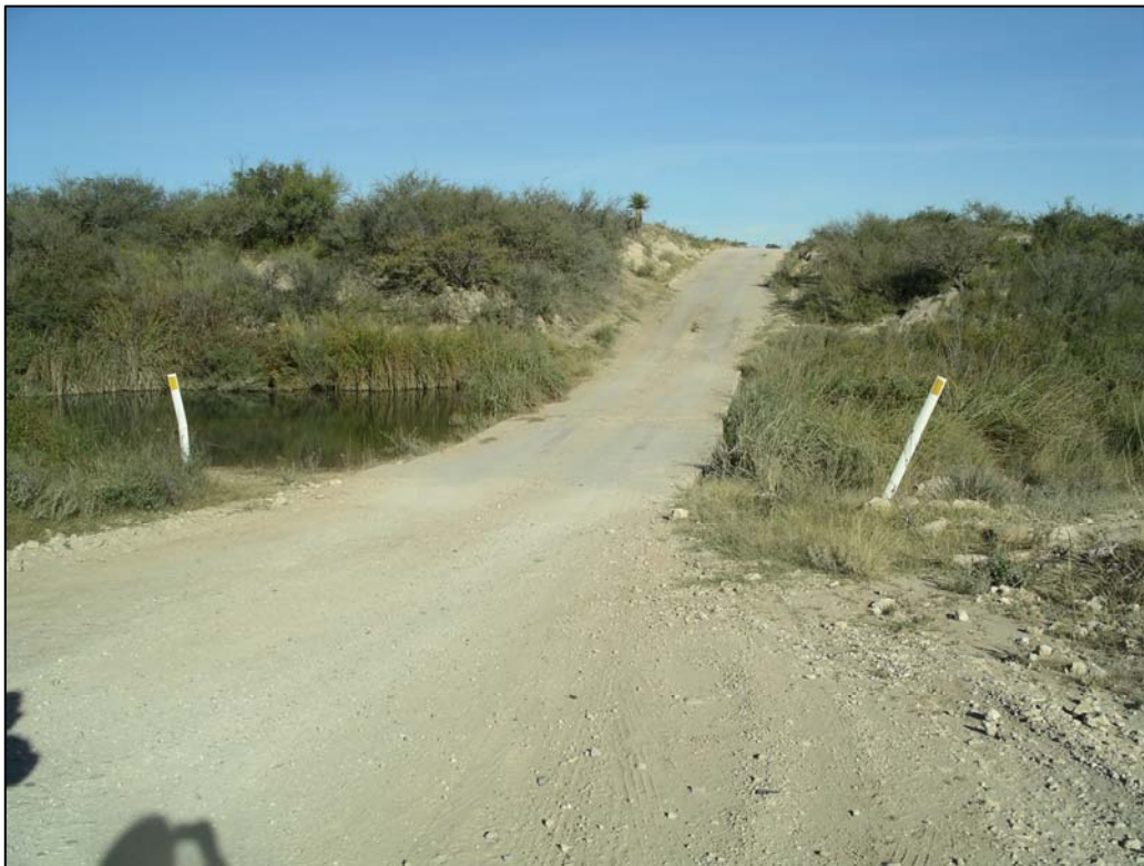
Figure 7. Low water crossing on the Black River, Eddy County, New Mexico. Photo: Julie McIntyr.
