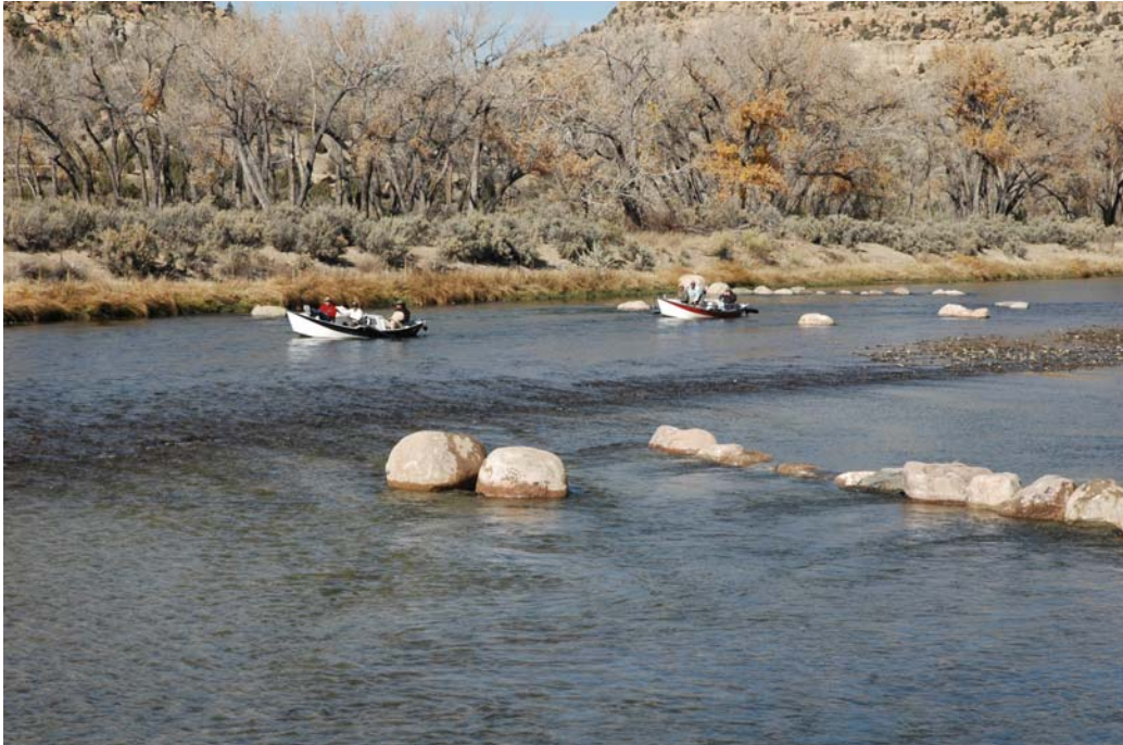
Figure 21. Example of a J-hook structure constructed as part of habitat enhancement projects in the San Juan tailwater.
