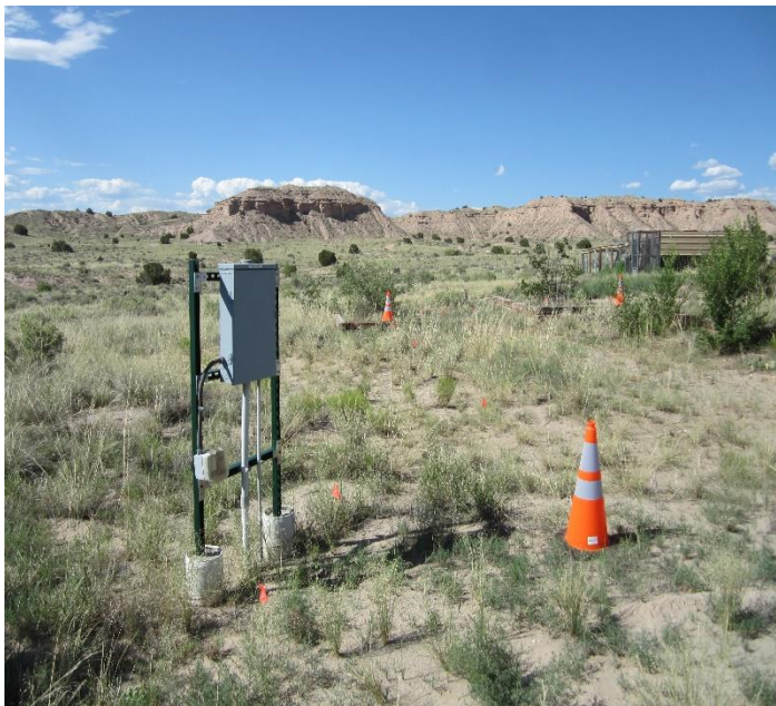
Electrical connection Southwest corner
