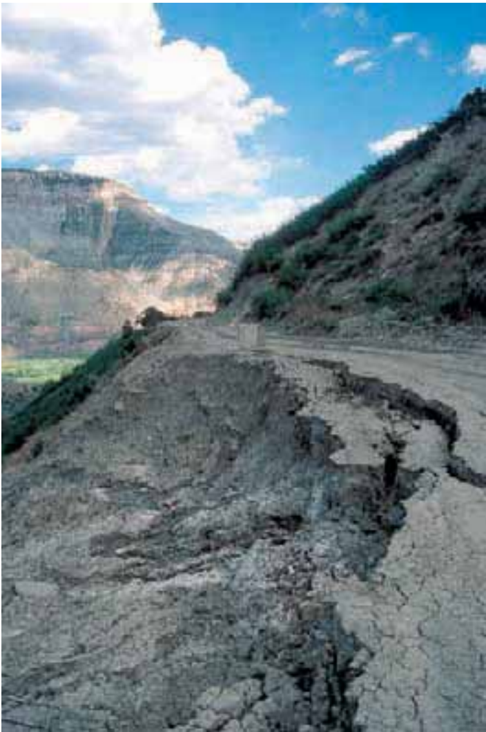
Figure 54. Erosion resulting from increased use and runoff. (Photo courtesy of CDOW).
