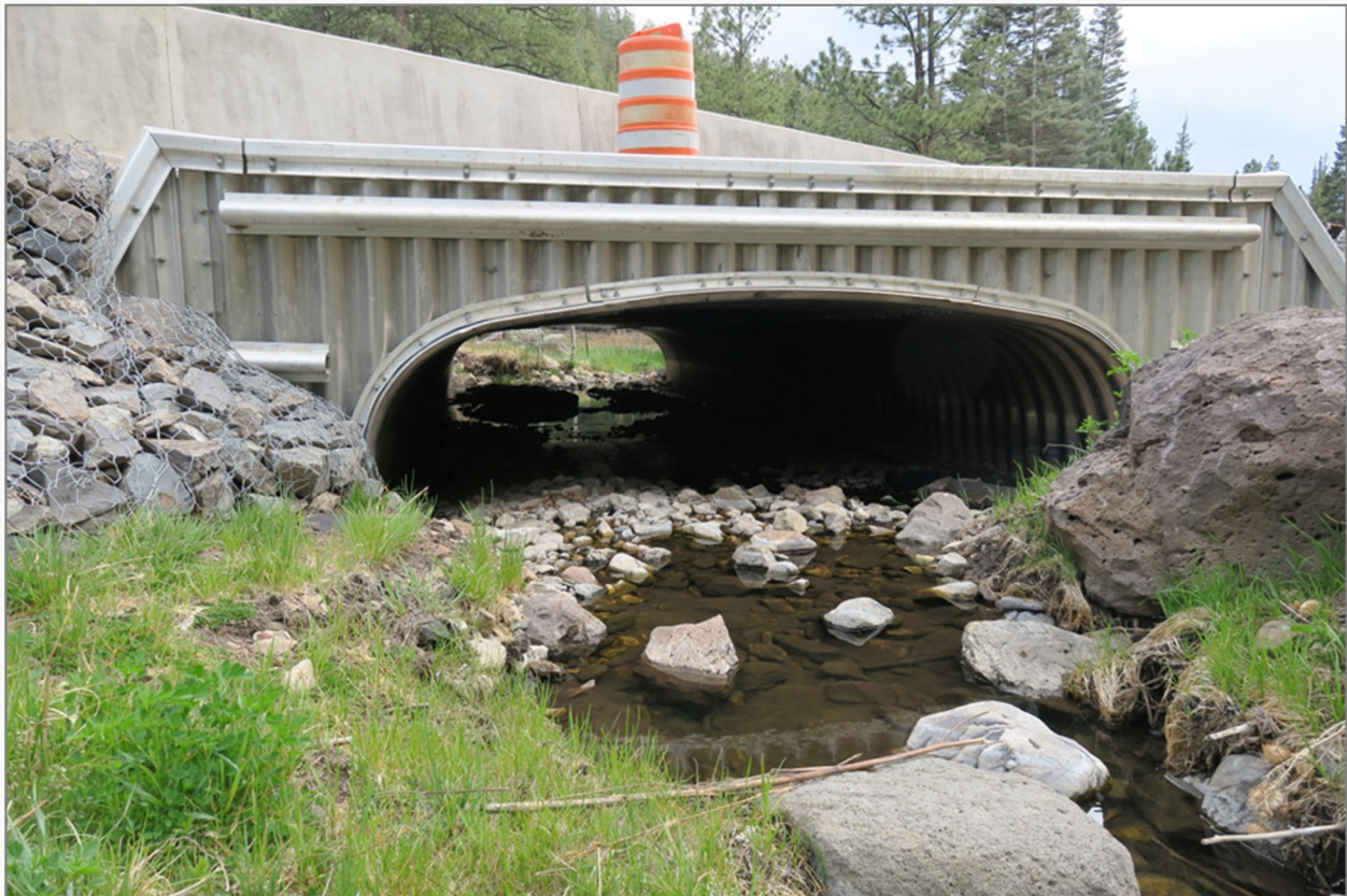
A successful bottomless arch culvert over Big Blue Creek (a tributary to Coyote Creek) along NM Highway 434 in northeast New Mexico. M. Volke .
