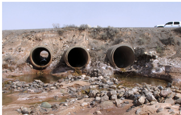
Low flow conditions along with improperly designed culverts block the movement of White Sands pupfish, a State Threatened species, at Holloman Air Force Base near Alamogordo. M. Watson.
