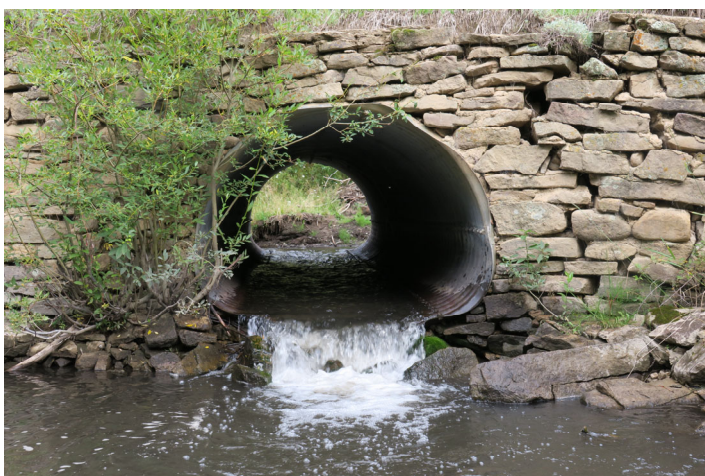
An abrupt drop at a culvert outlet restricts upstream animal movement. M. Volke.
