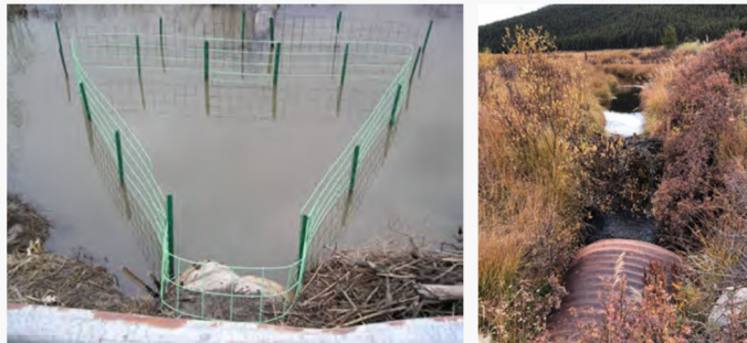
Left: An example of culvert fencing. S. Boyle . Right: Starter dam upstream of a culvert. P. Planer, RangeWorks LLC .
