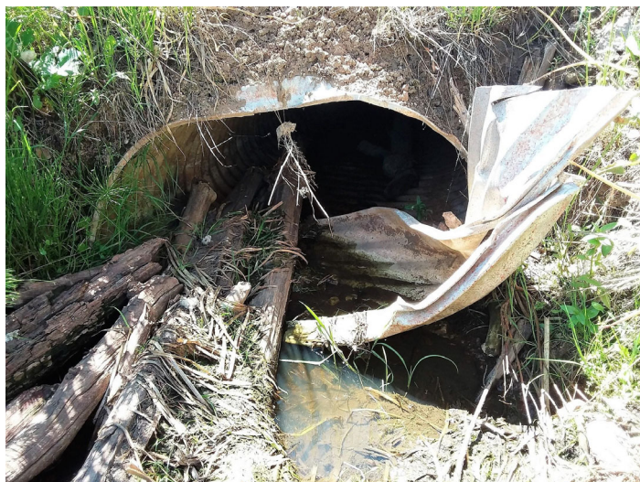
Debris accumulation at a culvert impedes animal movement. M. Volke.
