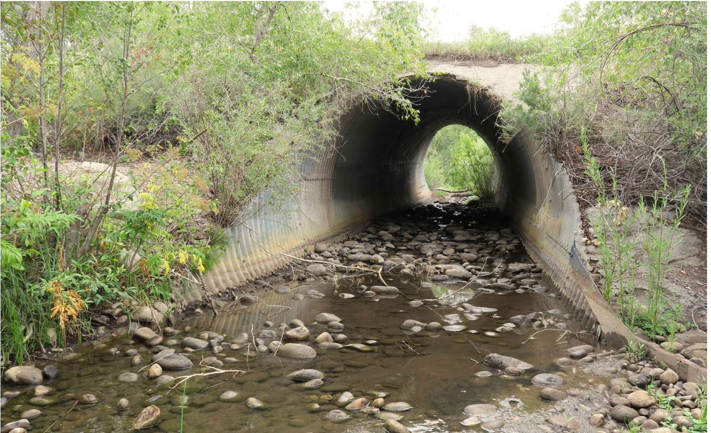
This large culvert provides a seamless transition between the natural stream and artificial structure, along with a natural substrate through the entire crossing, enabling aquatic life movement. M. Volke.
